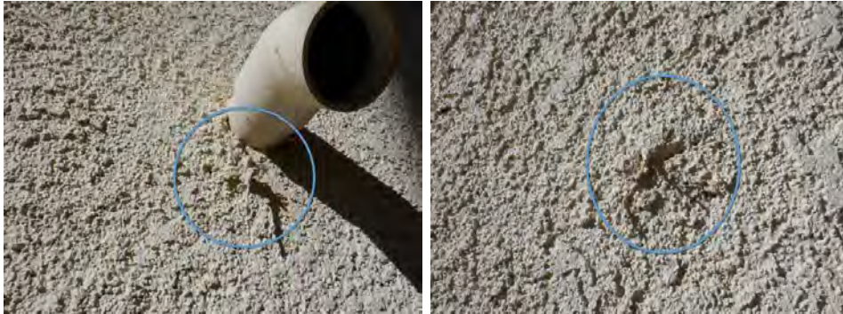
Two Feet Above Garage Occupant Door
