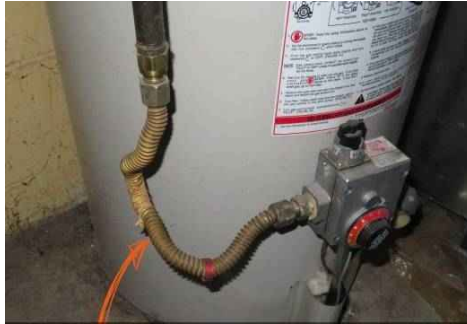
Example of (Outdated) Brass FAC which should be replaced
